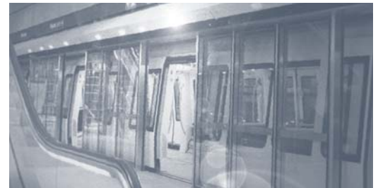
Seals on sliding platform screen doors
