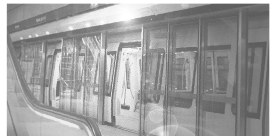
Seals on sliding platform screen doors
