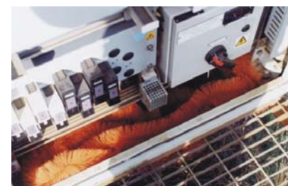
Guarding against rodent intrusion at the base of a trackside enclosure
